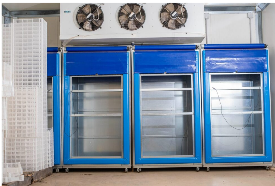
Figure 8: Cold storage facility for avocado export
